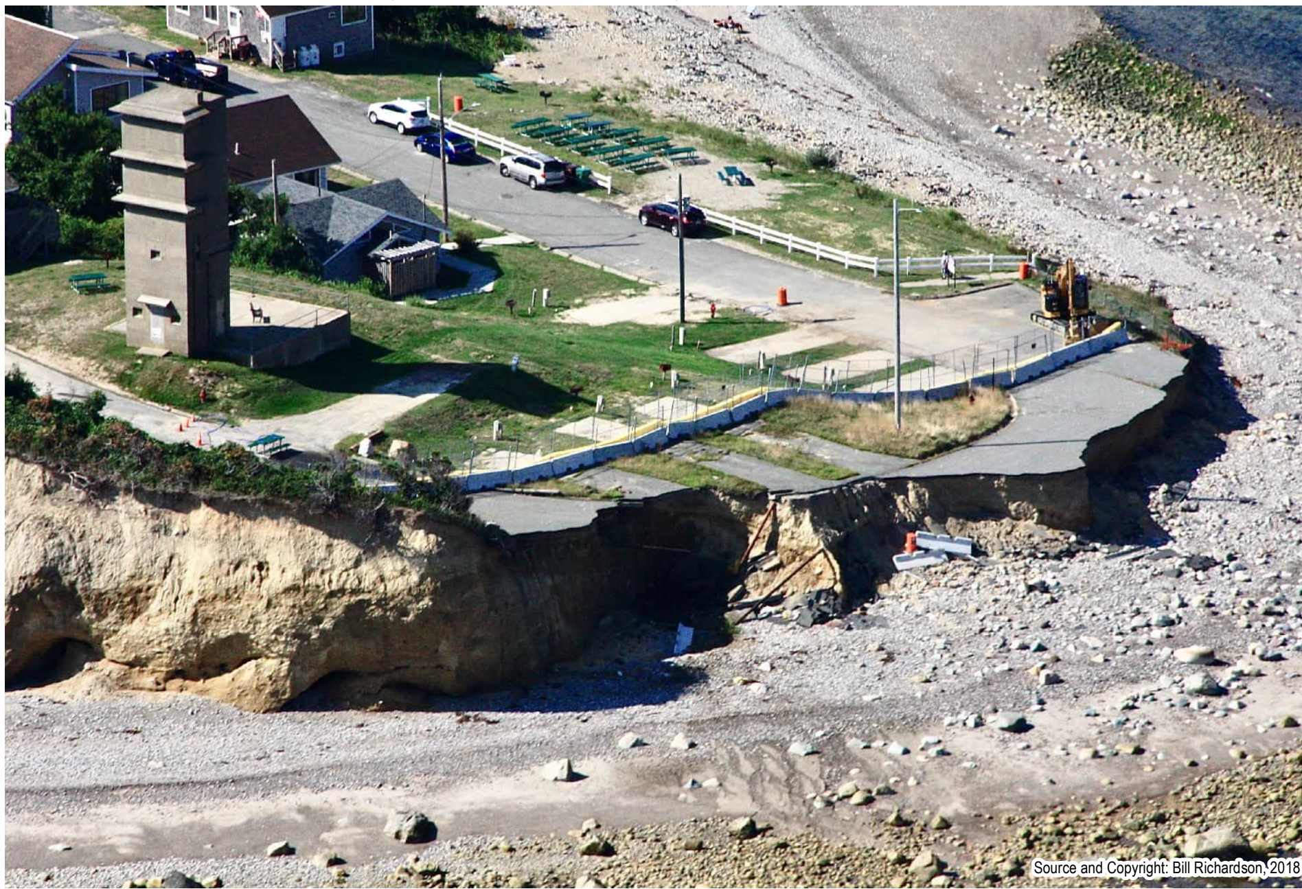
Figure 1-3: Fourth Cliff Existing Conditions-Toe Closeup
